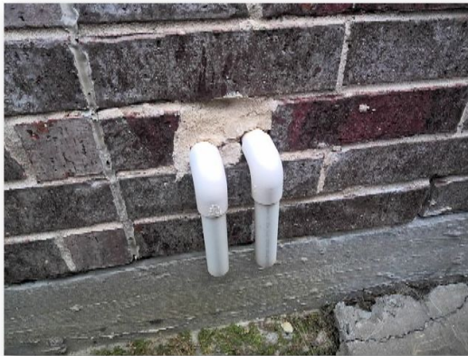
TPR Valve Drain Line
