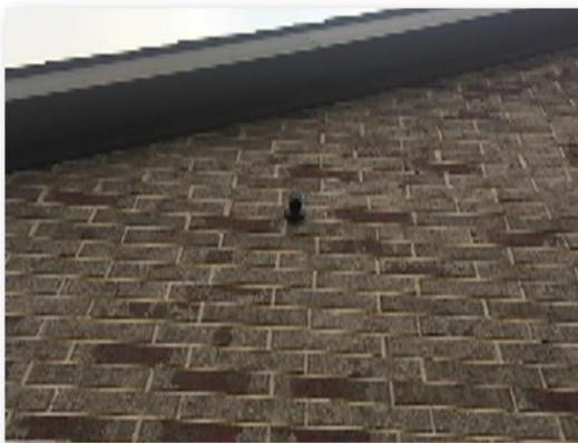
Secondary Drain Line
