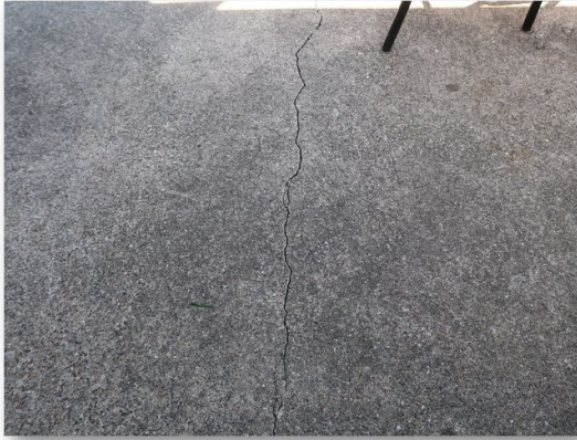
36. There are tile cracks and hairline cracks in the floors of the front porch and backyard patio.
