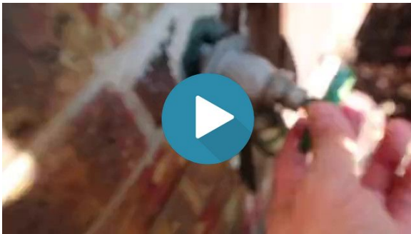
55. An exterior faucet near the front of the home was leaking.
