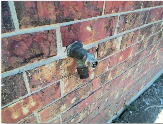
One of exterior faucet missing the handle.
