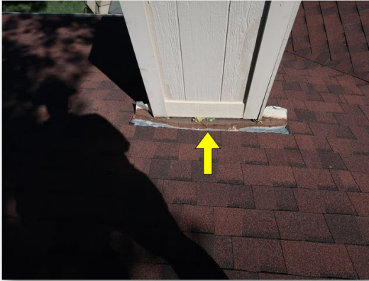
33. The chimney had no cricket.
