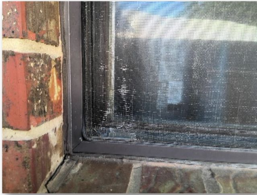
East wall Window screen was damaged
